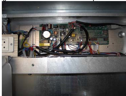
SWITCH REGULATOR BOARD and POWER BOARD
